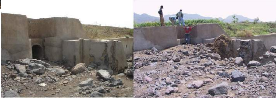
Pipe off-take at Tirke spate irrigation scheme before and after it was filled with sediment
