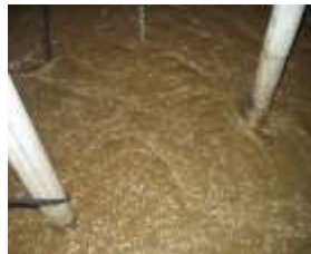
Aeration in biological treatment tank
